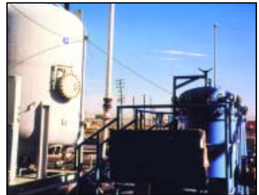
Fig 1. Storm water Cleanup system at a Refinery. 2000 gpm, 75,000 lb Oilsorb.
